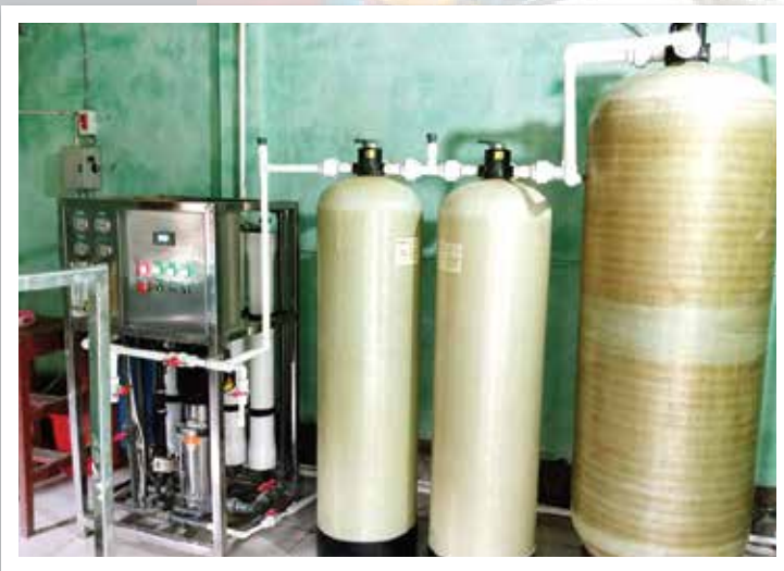
Desalination Plant at Nizlathimara village under Pathaoghata Upazila
